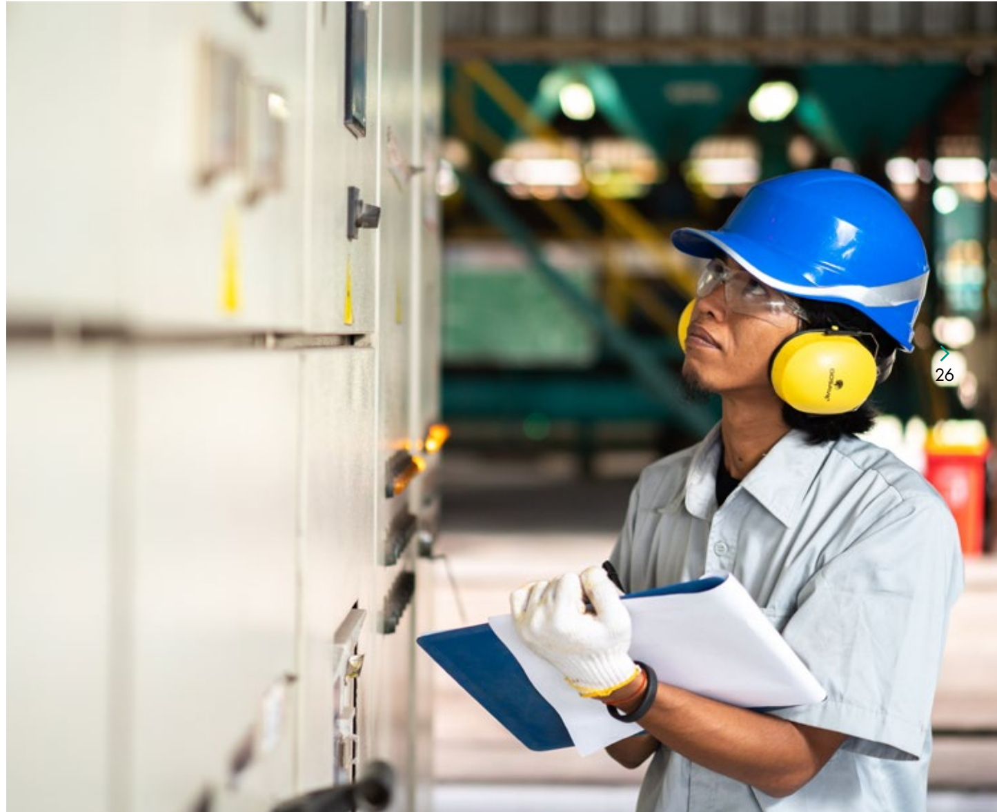
Energy consumption monitoring in our Cipta Graha POM, Kutai Timur, East Kalimantan
