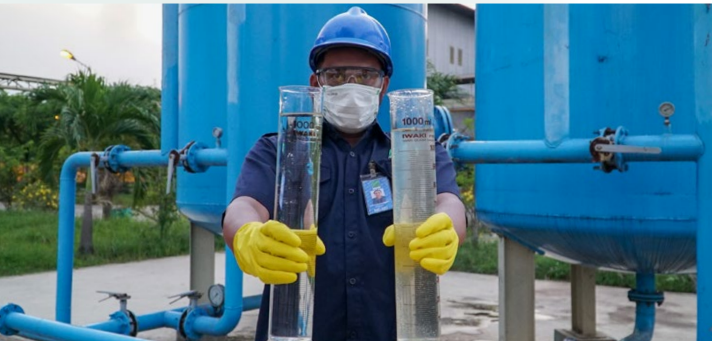
Water Treatment Plant in Arta Kencana POM, Lahat, South Sumatra
