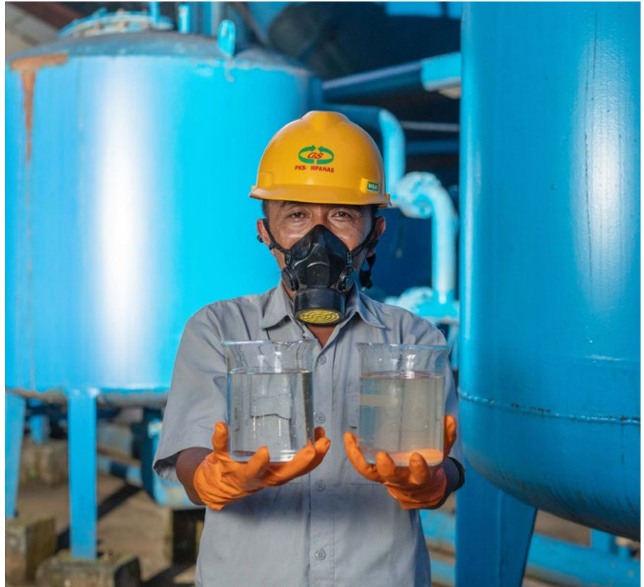
Water Treatment Plant in Ampanas POM, Kutai Timur, East Kalimantan
